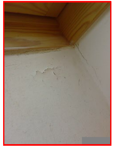
Bathroom Window Window frame/sill - peeling (lightly)
