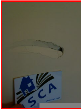
Living Room Wall Wall finish - dented (behind door)
